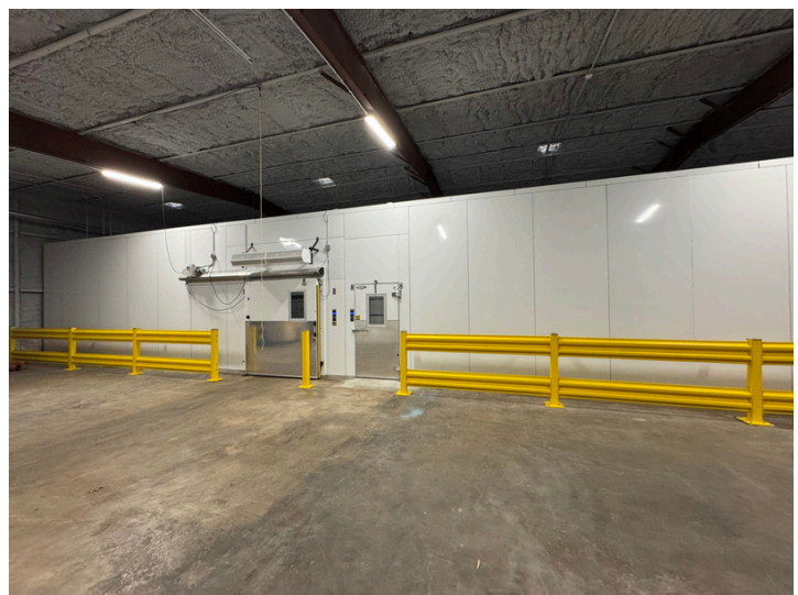
Annex Cooler Installed
